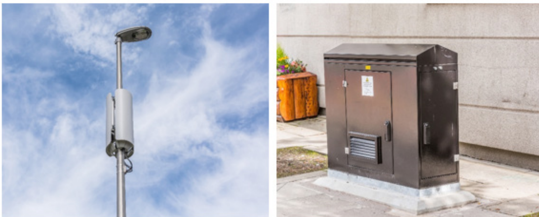
Figure 6: An example of a small cell antenna system and a street cabinet
